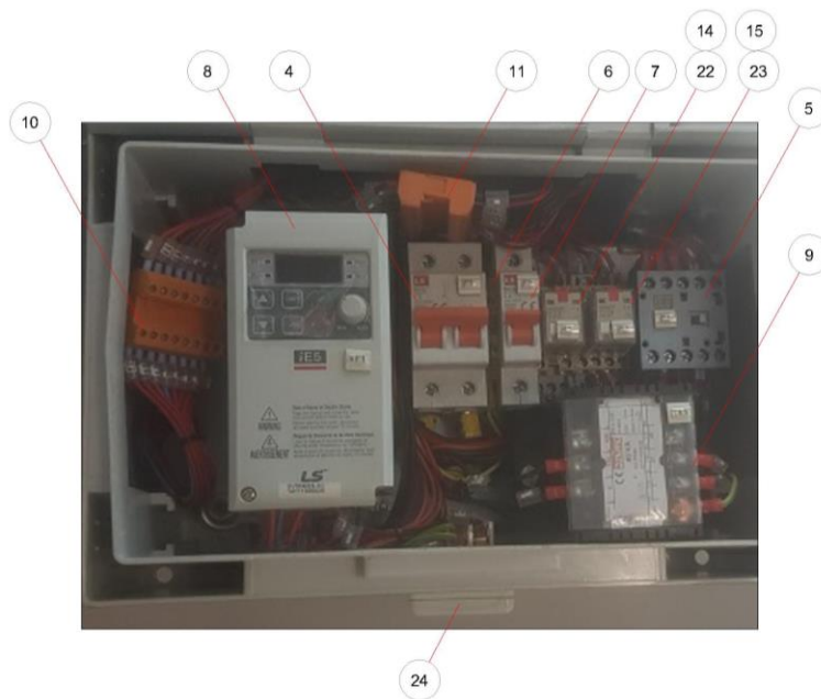
Figure 21. Electrical cabinet overview 1
