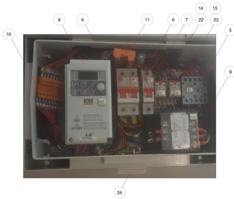
Figure 21. Electrical cabinet overview 1
